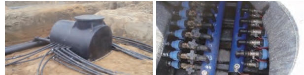
A ground heat exchanger pipe header
